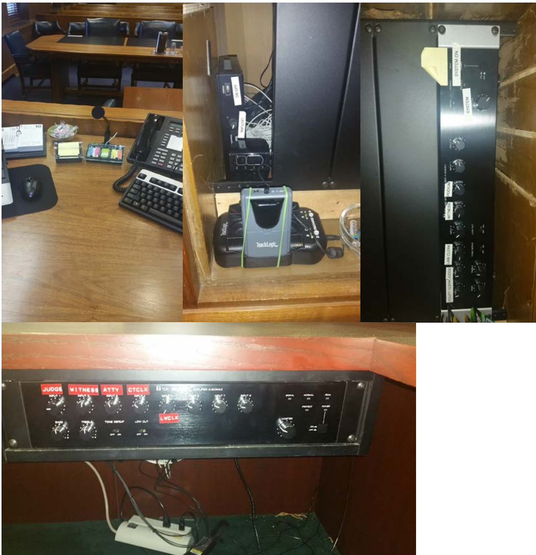
Figure 1: Photos of existing audio system.
